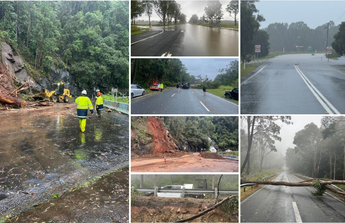
Figure 6. Emergency road management during ex-Tropical Cyclone Alfred
